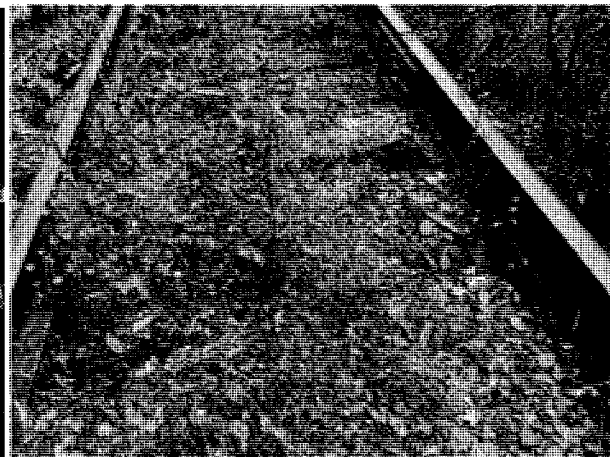
Photo 14 Fire damaged track and substandard ballast.
