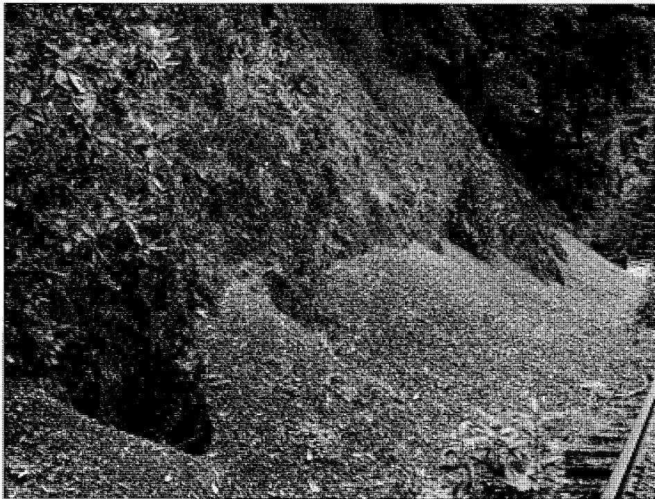
Exhibit 4-3 – Photo 65 – Fragments of highly fractured siltstone and mudstone raveling from rock slope at approx. MP 147.3
